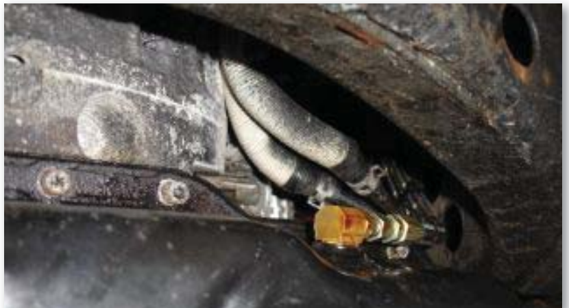
RETURN LINE TO TANK FLANGE.
