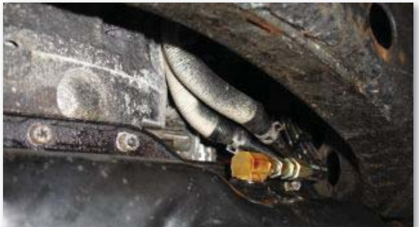
RETURN LINE TO TANK FLANGE.
